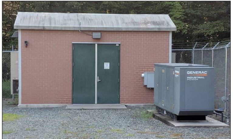
This building houses a pump station on Elizabeth Brady Road. A generator helps ensure it continues to operate, preventing spills.
